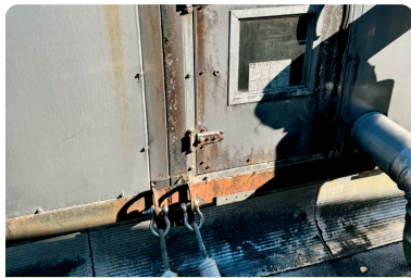
Salt water corrosion on a steel base
